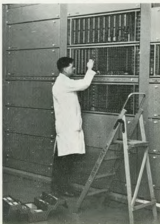
Mike Ellis ( foreman, Telecommunications ) adjusts one of the crossbar switches in the automatic exchange
