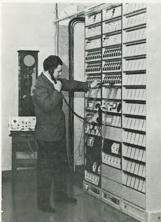
Brian Neild ( 2nd assistant engineer—Technical ) is shown here making tests on a telephone channel to Liverpool
